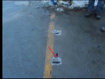
Screw drive penetration test indicating a de-tensioned PT tendon on the flat portion of the Roof Level
