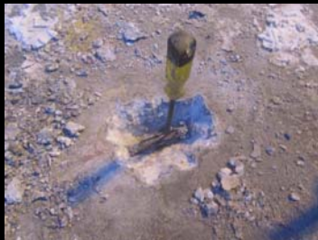
Screw drive penetration test indicating a de-tensioned PT tendon on the ramp at the Roof Level
