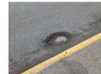
Photo 6: Hole in S02E in the P8E. Location: S02E in South of Pier 8 (Piers 8B to 8E).
