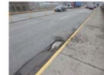
Photo 5: Large hole out of wheel path, concrete deck has been exposed. Location: S02E in South of Pier 8 (Piers 8B to 8E).
