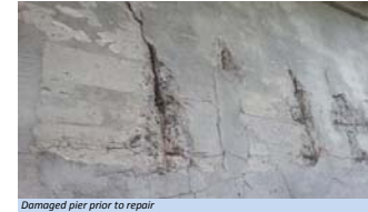
Damaged pier prior to repair
