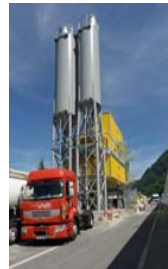
Portable batching plant; one silo for sand, one silo for the premix, 2 high shear mixers 1 m 3 (1.5 yd 3 ) batches
