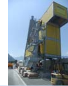
On site portable batching plant – 2 mixers
