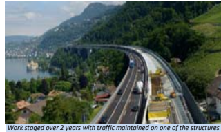
Work staged over 2 years with traffic maintained on one of the structures
