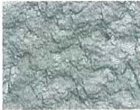
CSP 7 (heavy abrasive blast)
