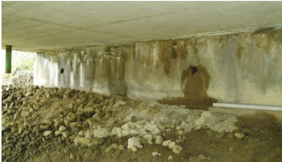
Fig. 1: Abutment condition prior to repair in May 2005
