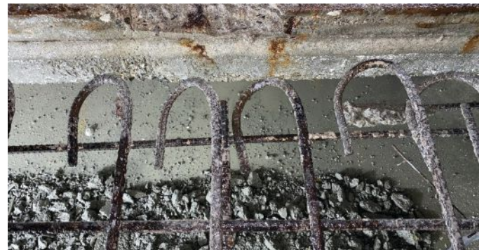
Fig. 5: Cement Paste Remaining on In-Situ Rebar
