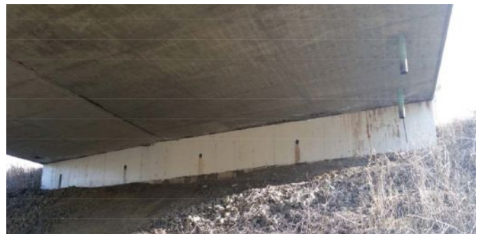
Fig. 10: Abutment of I-75 Bridge over Kirkwood Road (mm 87) in 2022 (Note efflorescence from leaking joint and weep holes)
