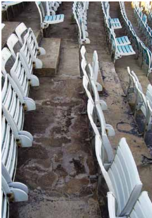
Corroded reinforcing steel resulted in spalling of the concrete—a significant hazard to patrons below
