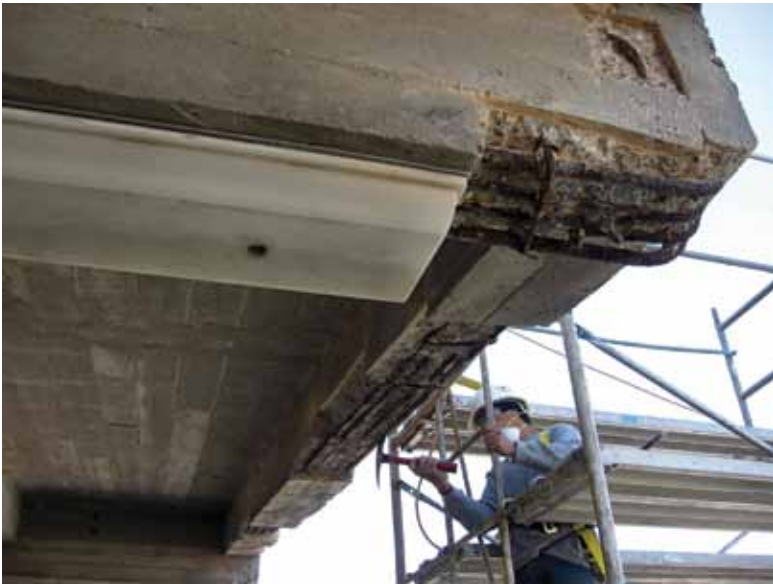
Sounding of concrete at underside of upper deck prior to installation of repair mortar
