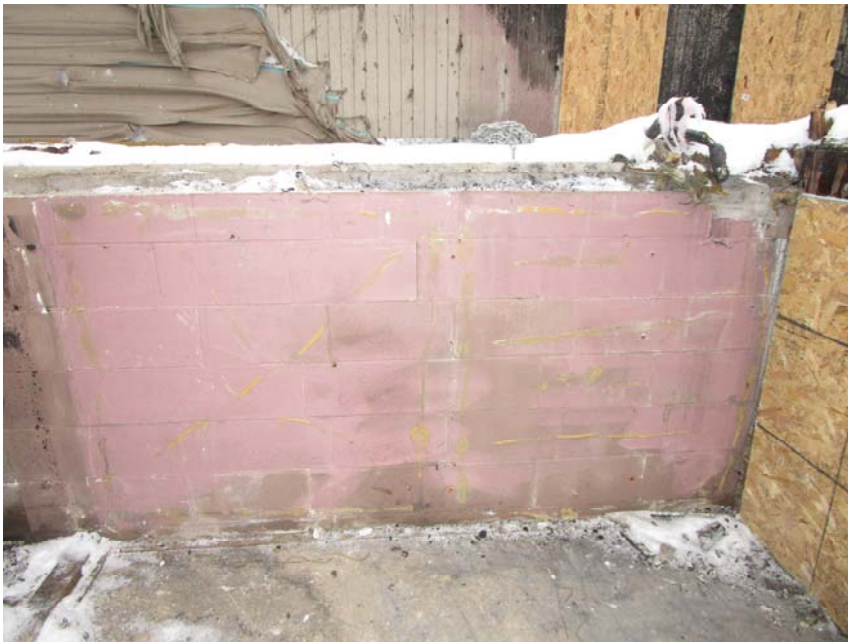
Painted surface with soot
