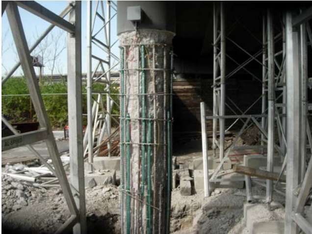
Bridge Column Jacket
