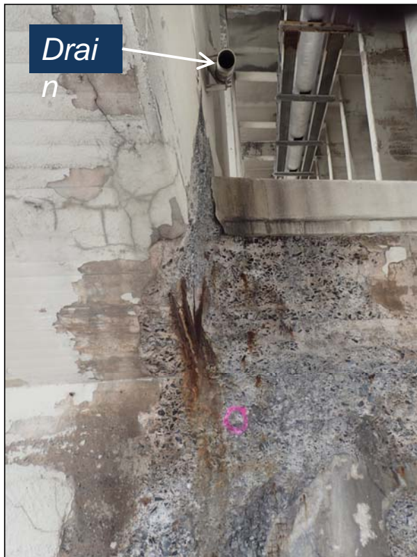
Deep F/T below drain
