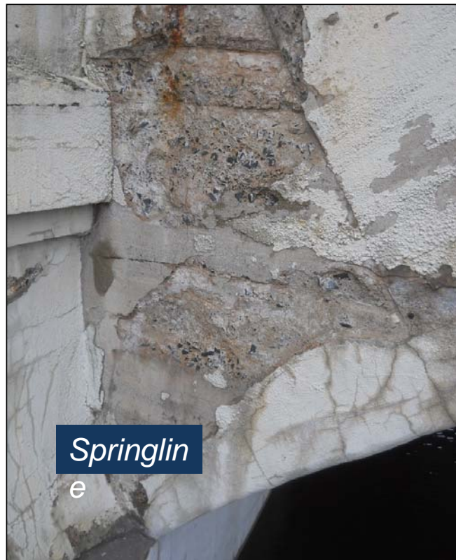
Deep F/T at arch springline
