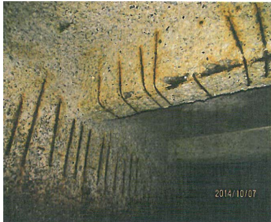
Credit: Daryl Prefontaine : Repair & Protection of Wastewater Infrastructure: Gold Bar Influent Channel No. 2, Concrete Repair Bulletin, 2016, ICRI
