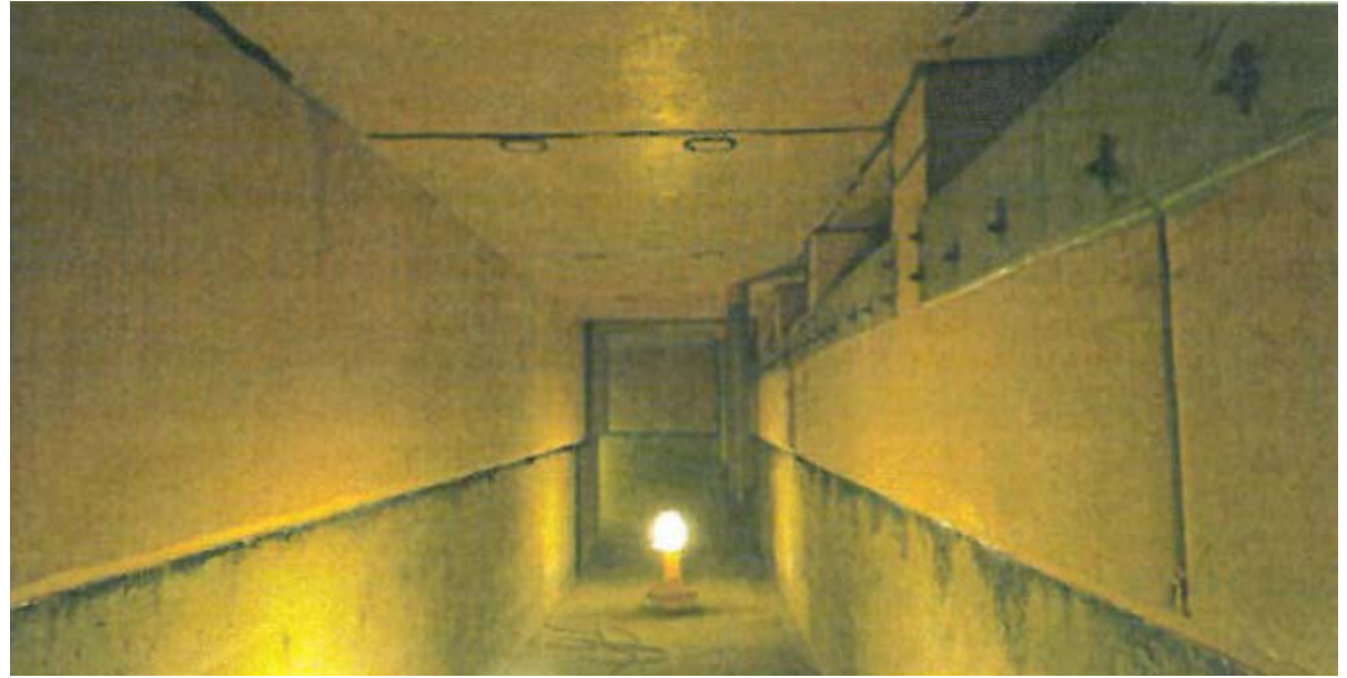
Credit: Daryl Prefontaine : Repair & Protection of Wastewater Infrastructure: Gold Bar Influent Channel No. 2, Concrete Repair Bulletin, 2016, ICRI
