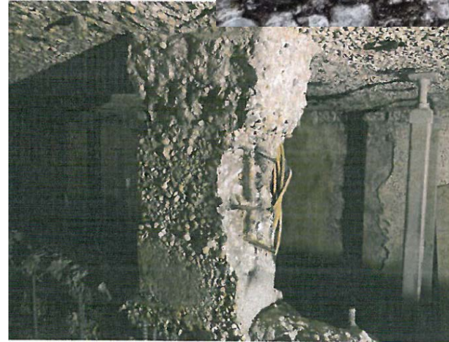
Credit: Daryl Prefontaine : Repair & Protection of Wastewater Infrastructure: Gold Bar Influent Channel No. 2, Concrete Repair Bulletin, 2016, ICRI
