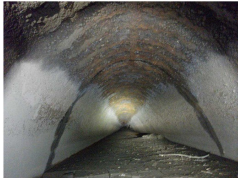
Photo 10: Example of hydrogen sulfide corrosion.
