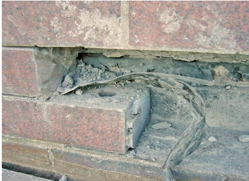
Fig.7 This wall has many inherent defects with the flashing and cavity wall drainage
