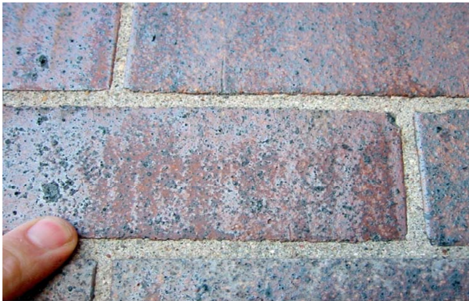
Fig. 12 Example of surface coating entrapping water beneath the coating
