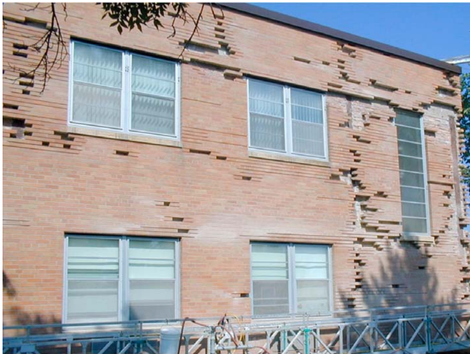
Fig. 2 This wall was repaired twice, after the roof leaked for many years
