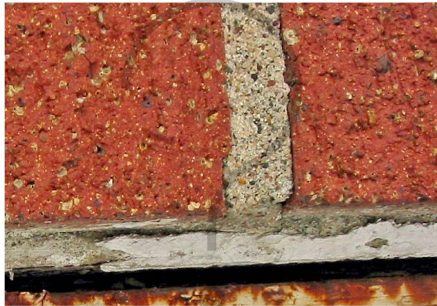
Fig. 1 Shelf angle sealed at front edge preventing water drainage
