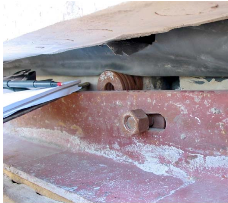
Fig. 17 The shelf angle is shimmed with haphazardly placed washers
