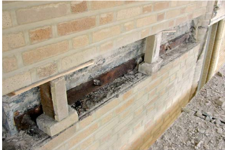
Fig. 5 Existing shelf angles were left in place, even though there was no through-wall flashing or other protection
