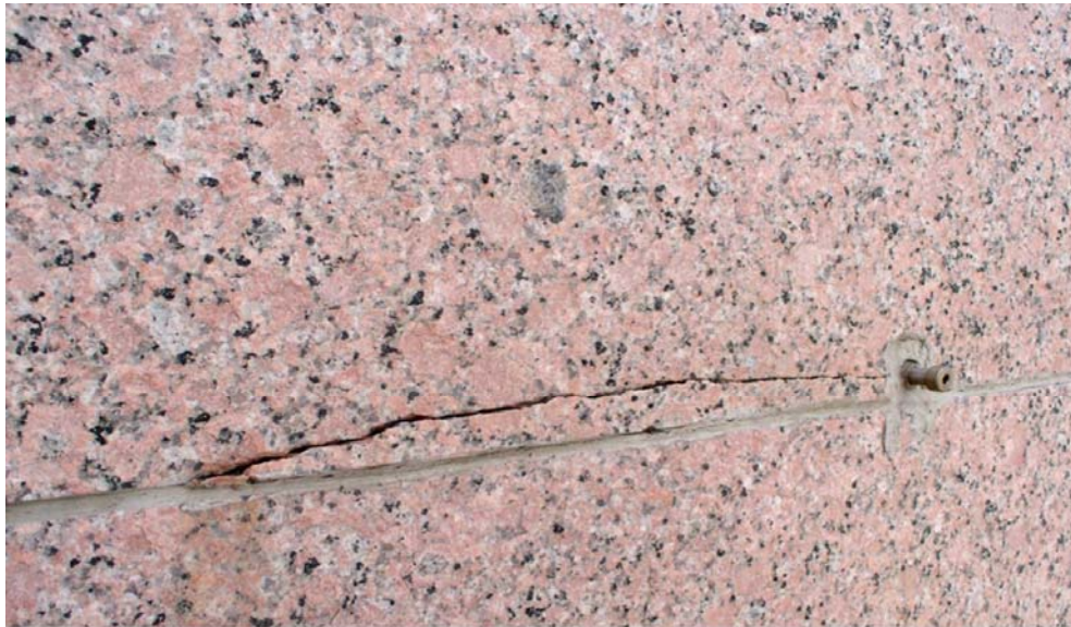
Fig. 9 Cracked stone panel at horizontal joint. Note lack of weeps in joint
