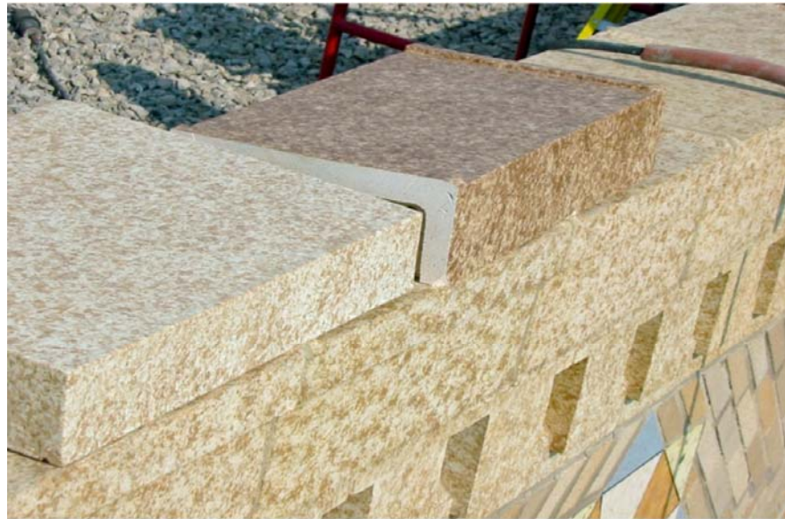
Fig. 4 Matching terra-cotta was a time-consuming, exacting process. Note the too-dark mockup piece on the right.
