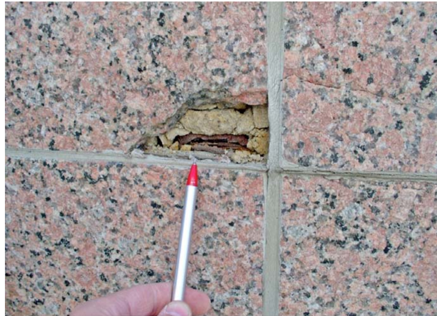
Fig. 11 (Color online) Spalled stone corner reveals corroded support
