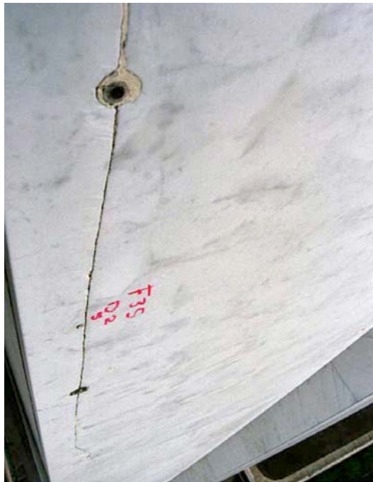
Fig. 15 Corner restraint at Carrera marble panel has a repair that has also failed
