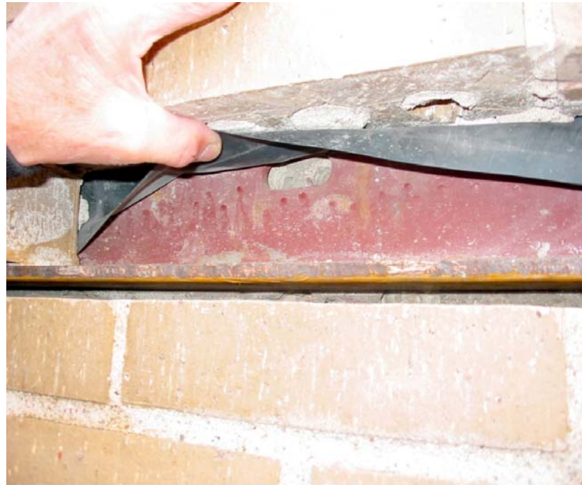
Fig. 16 Missing anchor at shelf angle
