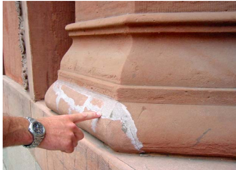
Fig. 13 Stone matching material has weathered poorly and is incompatible with the parent brownstone
