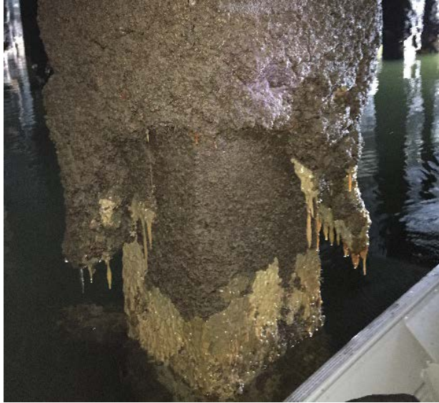
Pile Jacket Deterioration
