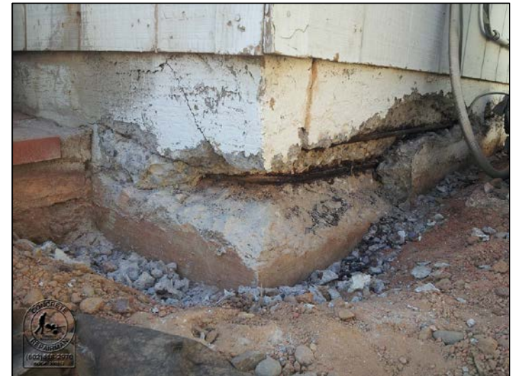
Temperature & Moisture Deterioration
