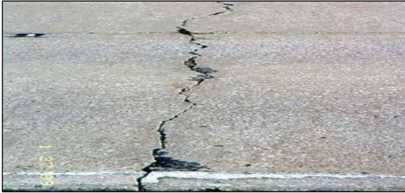
Thermal Stress Cracking
