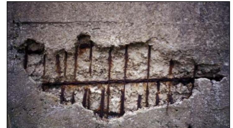
Spalling caused by Corrosion of the Steel Reinforcement
