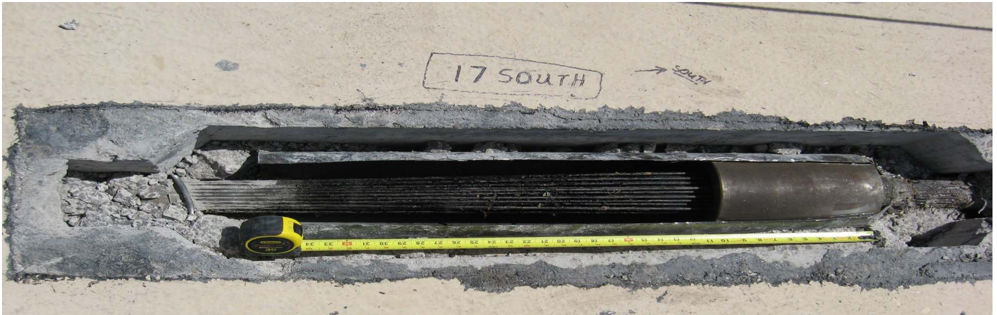
Photo #3 (above) shows cable coupling in normal position, with straight parallel wires. This occurred at the un-failed end.
