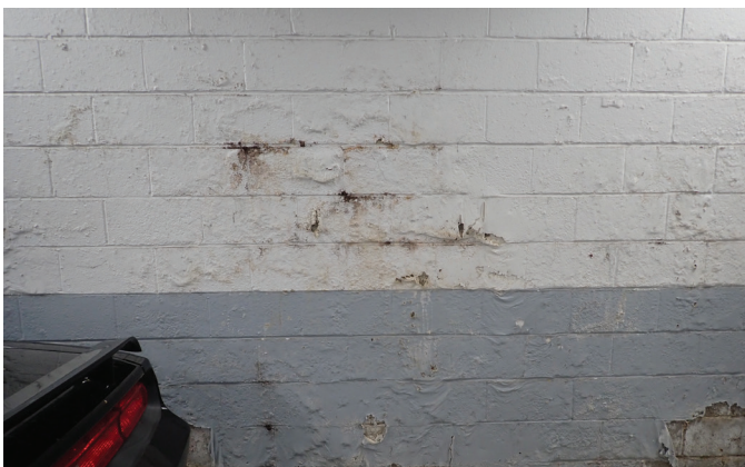
Fig. 1: Water intrusion through CMU wall before grout injection (Picture courtesy of Martin/Martin Consulting)
