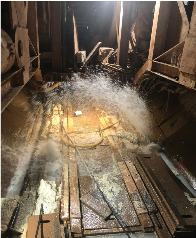
Fig. 6: High-pressure water leakage in a tunnel boring machine (TBM) underground
