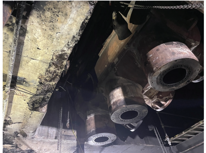
Fig. 4: Deep spalling with exposed reinforcing along edge of equipment penetration (marked with red arrow)
