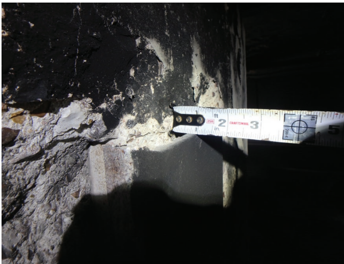
Fig. 6: Typical damage to embedded channels. Channel is pulled away from the surface of the concrete by approximately one inch
