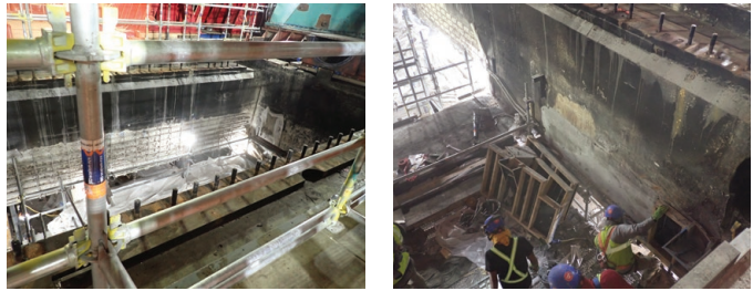
Fig. 13: Vertical concrete repairs on face of equipment penetration during demo (left) and during formwork removal (right).
