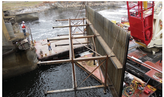
Fig. 2: Downstream dewatering using surface skin plate, supported by custom steel frame support system
