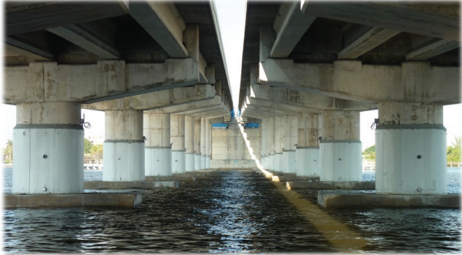
Fig. 3: Galvanic jacketing to protect bridge columns in a marine environment. The jacketing system includes alkali-activated distributed anodes inside stay-in-place FRP formwork
