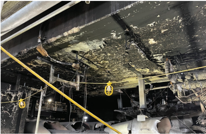
Fig. 1: Fire damage to turbine pedestal and piping, photo taken a few days after fire
