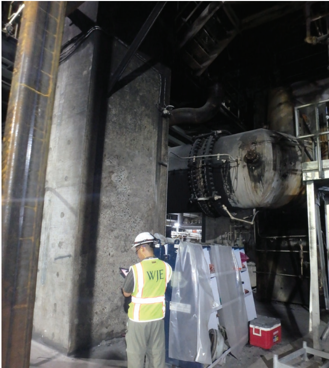
Fig. 5: Spalling on side of column
