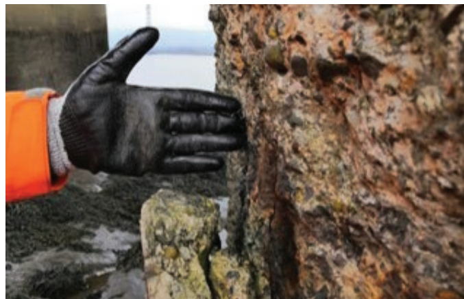
Fig. 5: Concrete deterioration in marine environment due to corrosion
