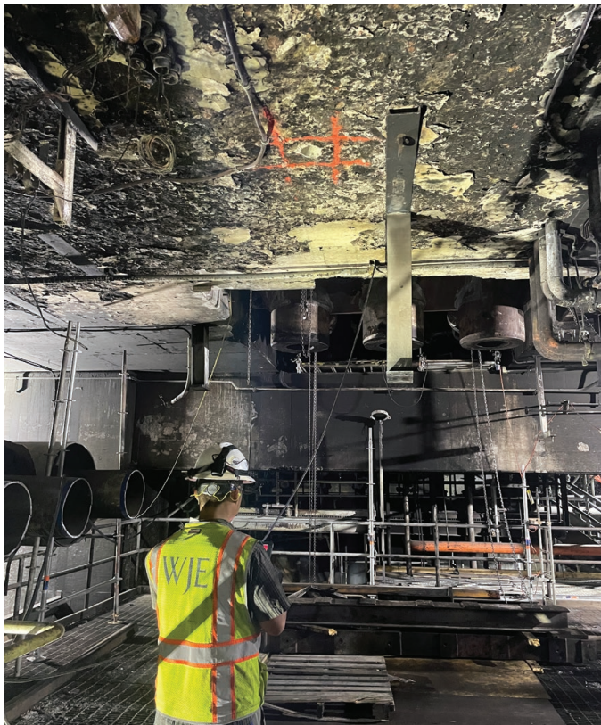
Fig. 3: Fire damage to soffit of upper deck. Extensive spalling is visible
