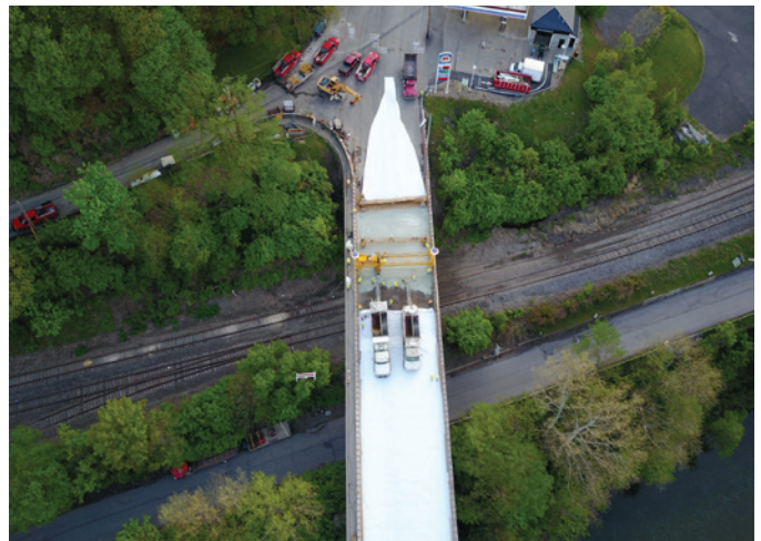
Fig. 4 A & B: The Thornburg Bridge’s reinforced concrete bridge deck was restored and preserved with a very early strength LMC (VESLMC) overlay. The smoothed surface was covered with burlap, hosed down, and covered with polyethylene plastic sheeting to cure for at least three hours
