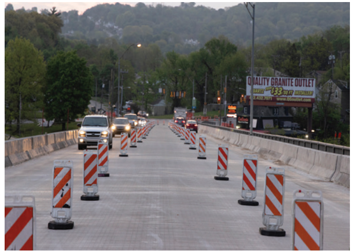
Fig. 7 A & B: The finished product: A very-early-strength latex-modified concrete (VESLMC) overlay that can be reopened to traffic after three hours
