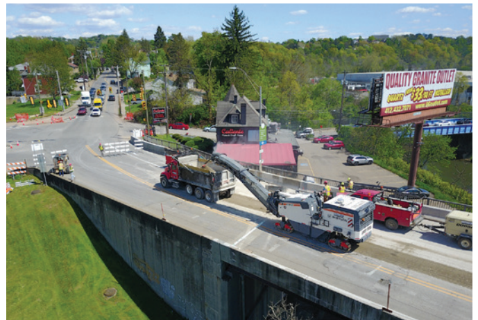
Fig. 1: The first step in placing any latex-modified concrete (LMC) overlay is removing the top layer of existing concrete. A cold-milling machine removed about ½ inch from the Thornburg Bridge deck in Pennsylvania via scarification
