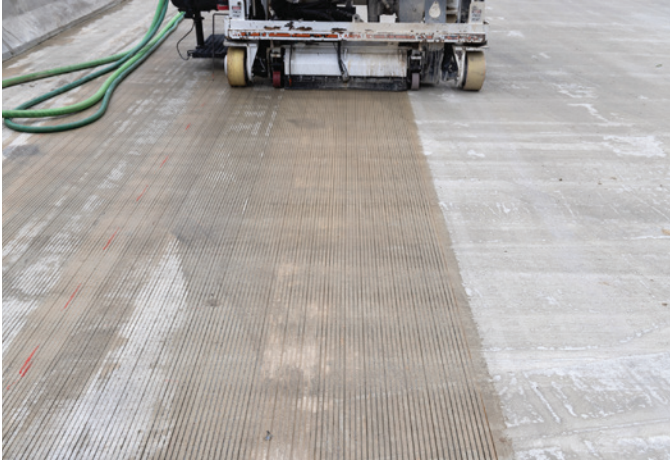
Fig. 5: After cure, the next step was texturing the very-early-strength latex-modified concrete VESLMC) overlay to increase friction and decrease noise. Like many state and local transportation departments, Pennsylvania DOT had the surface grooved longitudinally
