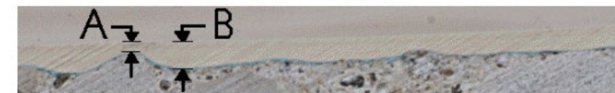
Thick, soft coating on concrete
