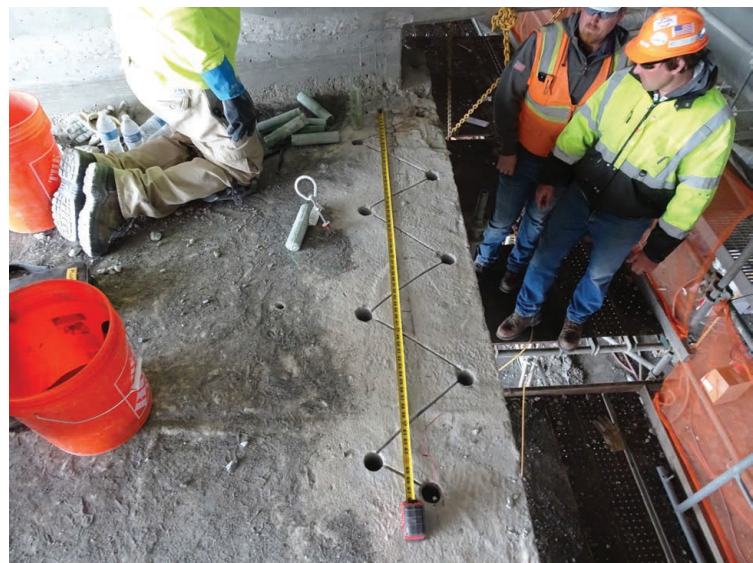
Image 11: Discrete, two-stage anodes installed in cored holes along sound arch corners between corner repairs
