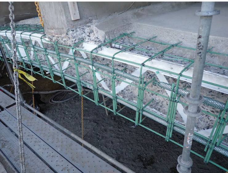
Image 7: Arch corner repair extending across full height of barrel arch, showing continuous and discrete CP anodes, supplemental rebar/anchorage, and coated Melan steel
