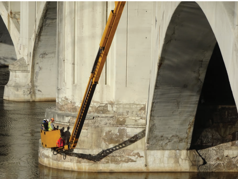
Image 3: Close-up inspection, illustrating deterioration in pier bases and arch ribs
