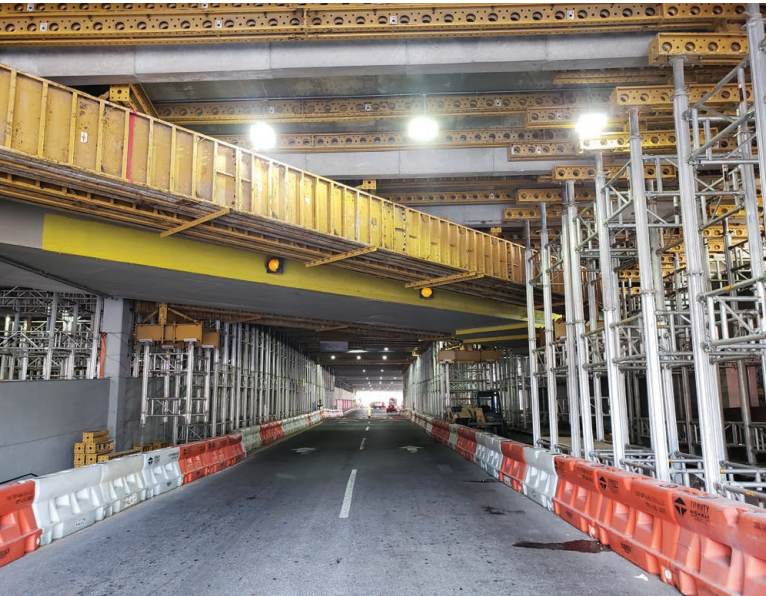
Shoring layout on Terminal Parkway to maintain partial use of the roadway during construction
