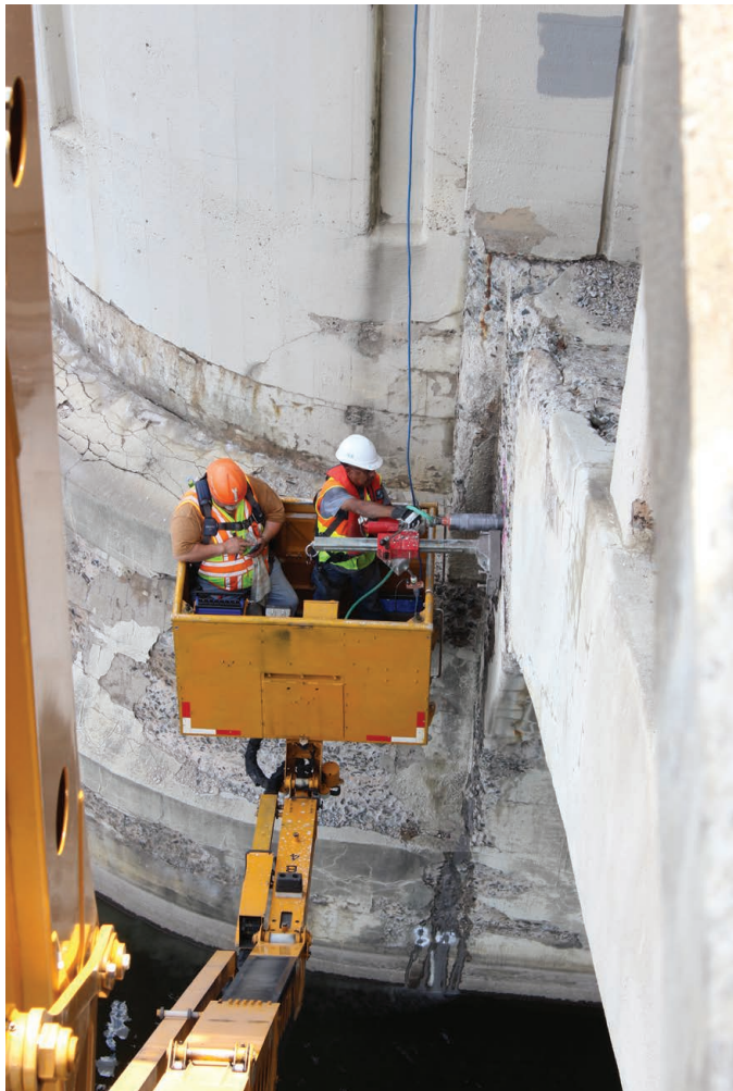
Image 4: Core sampling through deep freeze-thaw damage in arch rib near springline
