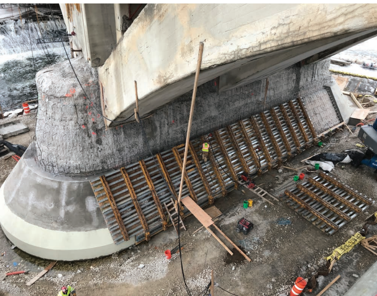
Image 9: Pier base jacket repair in progress, showing cofferdam, concrete removals, and supplemental rebar/anchorages at top, and formwork and new concrete jacket at bottom of pier
