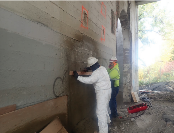
Image 12: Hand-finishing board form lines in shotcrete repairs on pier face to match existing surface texture
