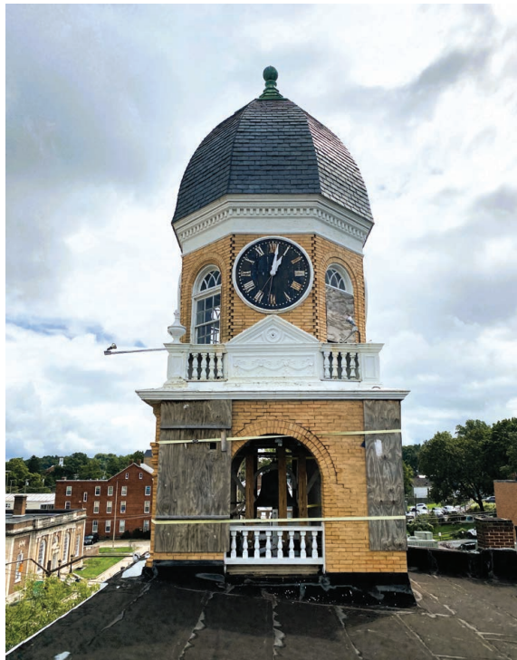
Image 2: Deficiencies in the tower base
