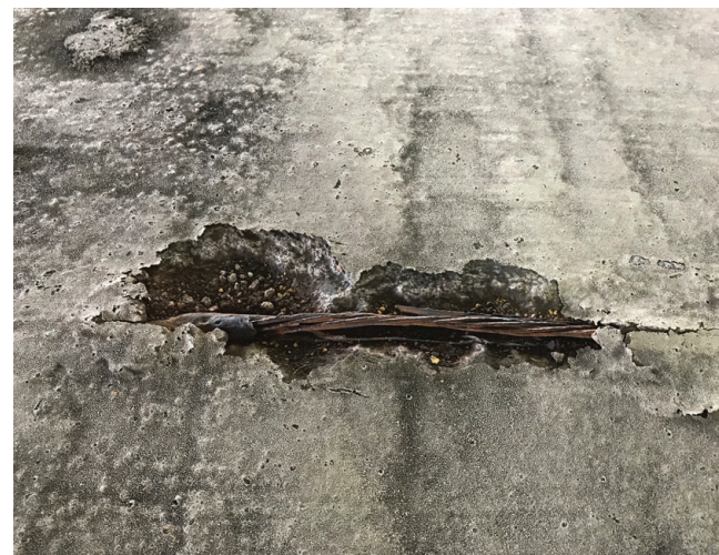
Failed PT tendon with multiple broken wires protruding from the top of the slab
