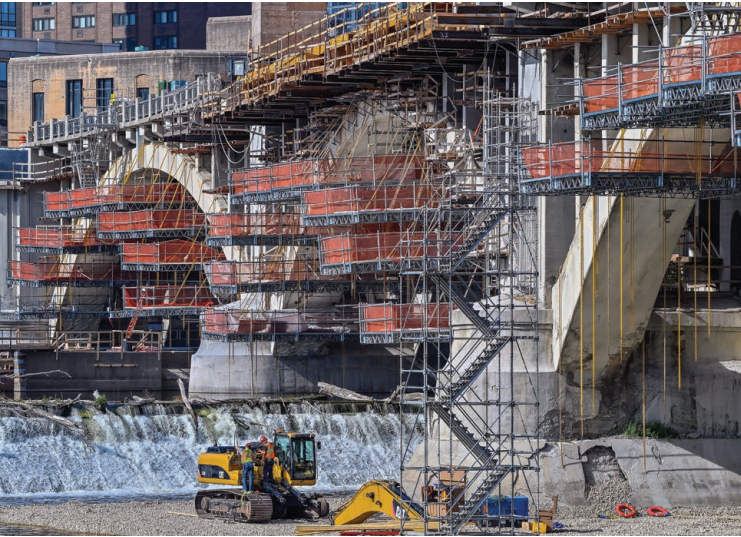
Image 6: View of multiple means of access, including suspended scaffolding and dewatered cofferdam. (Photo credit: Joe Szurszewski Photography)
