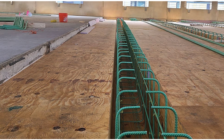
Image 9: Partial rebar detail with formed repair
