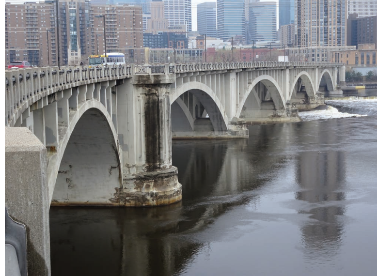
Image 13: "Before" photograph along upstream side of bridge, showing concrete deterioration in pier bases and arches
