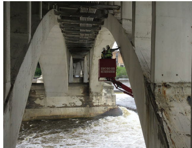
Image 2: Hands-on inspection from under-bridge inspection unit (snooper), illustrating deterioration of arch ribs and pier bases
