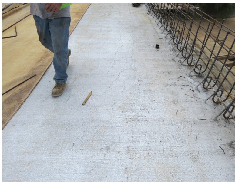
Fig. 2: Longer plastic shrinkage cracks running parallel to each other
