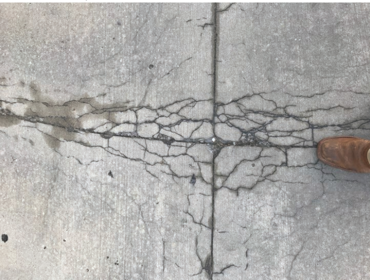
Fig. 5: “D-Cracking” at or near pavement joints
