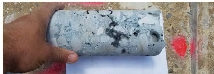
Fig. 7: Core 3—Darker, black sections indicate filling with epoxy resin
