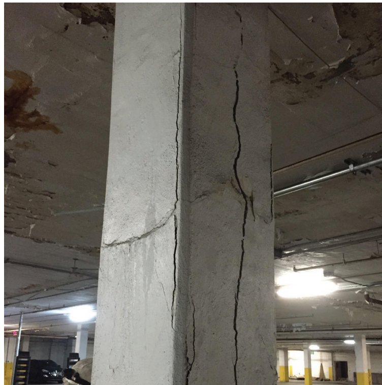
Fig. 9: Cracking with no rust staining present; could be indicative of structural cracking
