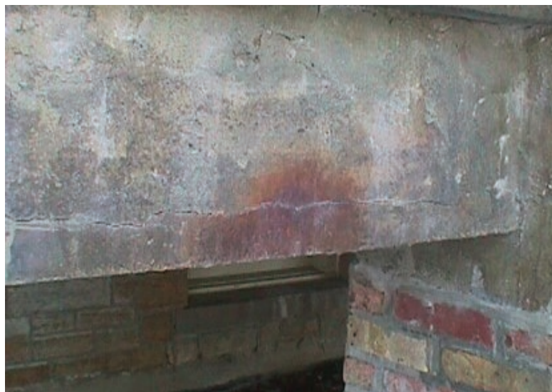
Fig. 7: Rust staining at cracks is an indicator that cracking may be due to corrosion of reinforcing steel within
