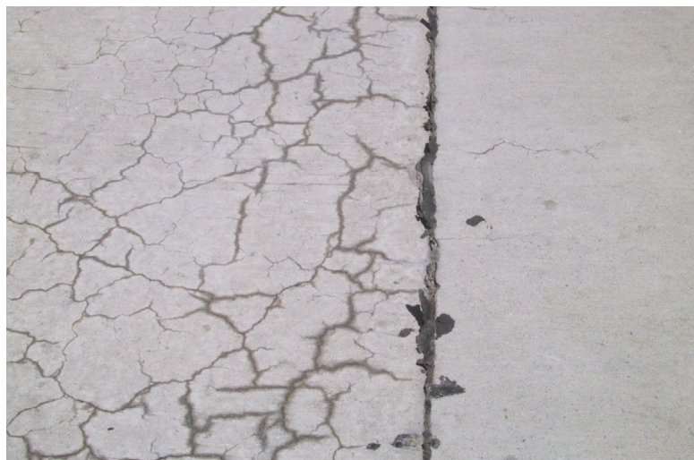
Fig. 6: ASR Cracking in distinctive Y pattern (FHWA) 15
