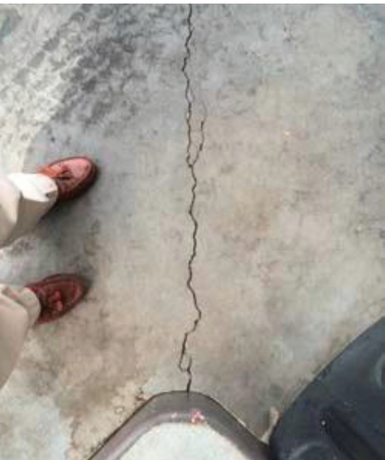
Fig. 3: Cracking is common at reentrant corners in concrete
