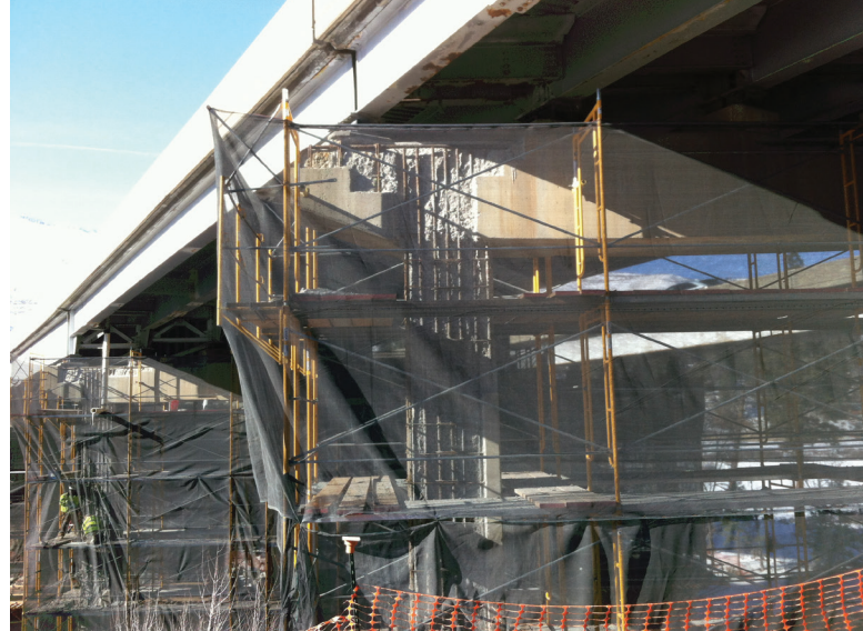
Figure 8: I-80 Verdi Bridge, Nevada, showing cut concrete and exposed rebar prior to repair mortar application (image courtesy of MAPEI).
