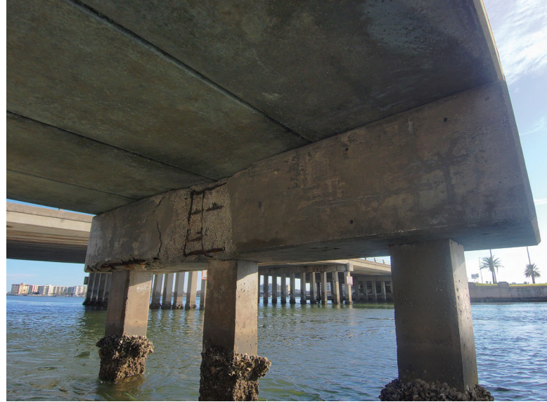
Figure 2: Bridge 1 Pier cap showing spalling and exposed corroded steel reinforcement
