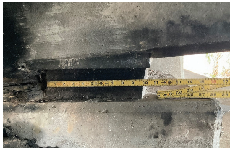
Figure 3: Bridge 2 North abutment shows bearings contracted \frac{1}{2} " to the South
