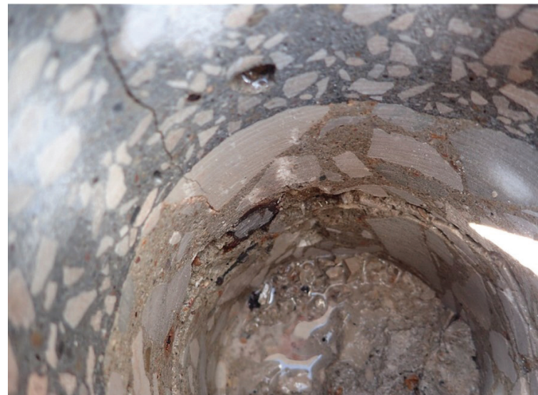
Fig. 3b: Corroded, embedded rebar with adjacent corrosion-induced cracking
