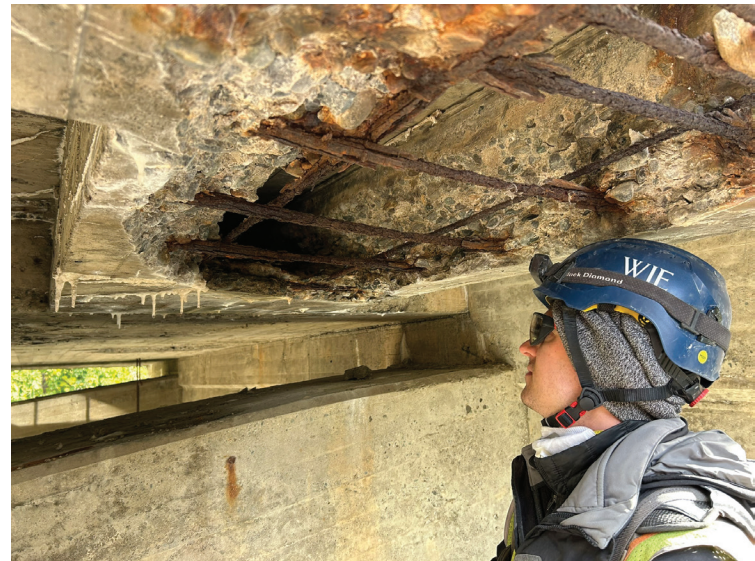
Fig. 3a: Example of corrosion in reinforced concrete; corrosion and spalling near drain
