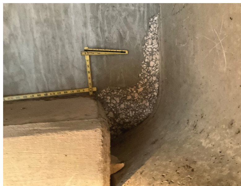
Figure 4: Bridge 2 South abutment, showing concrete spalling
