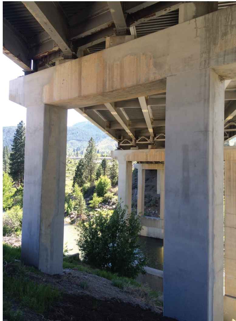
Fig. 9: I-80 Verdi Bridge, Nevada, showing cementitious fiber-reinforced, fluid mortar for formed repair (image courtesy of MAPEI).
